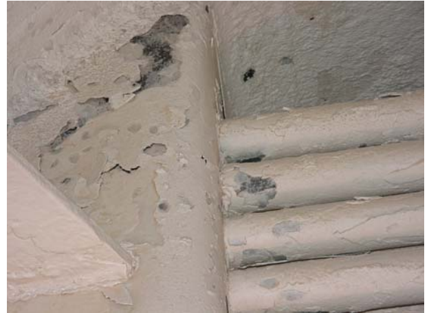
A light grey, soft scale layer was formed in boiler side
