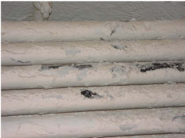
Scale on flame pipes is soft and easy to clean
