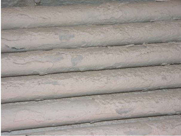
A light grey, soft scale layer adheres on the surface of the flame pipes
