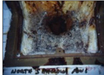
5 Rust disappeared. September 9, 1995
