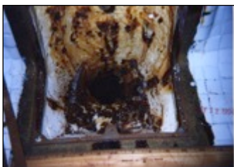
2 Rust problem. May 12, 1994
